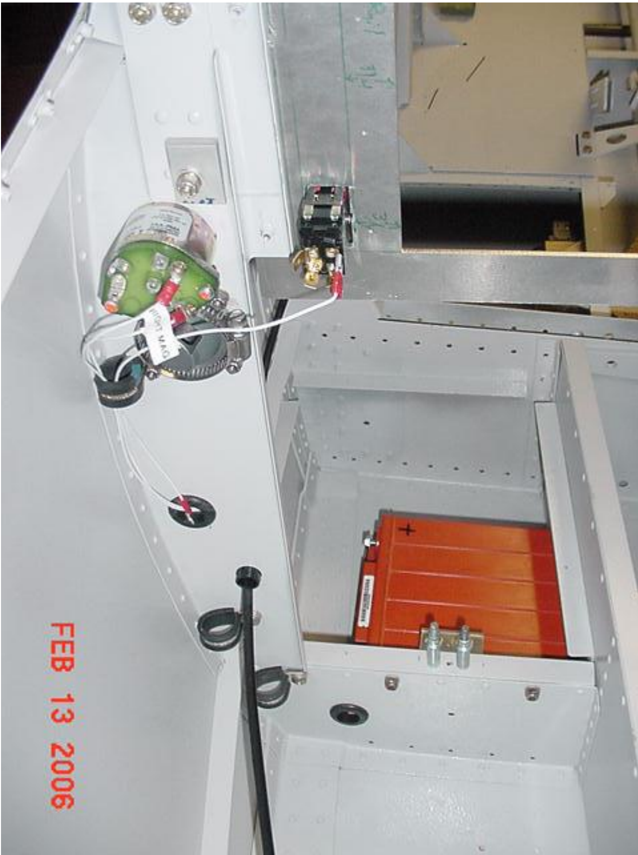
The primary positive power #4 AWG wires go from the primary battery to the "BAT" side of the primary battery solenoid, then branches out from the supply or "line" stud of the battery solenoid. An 8 AWG wire makes a short run to the Main bus (which is just a Blue Sea DualBus terminal strip near the rocker breakers behind the left instrument panel). A separate 4 AWG wire goes from the line side
