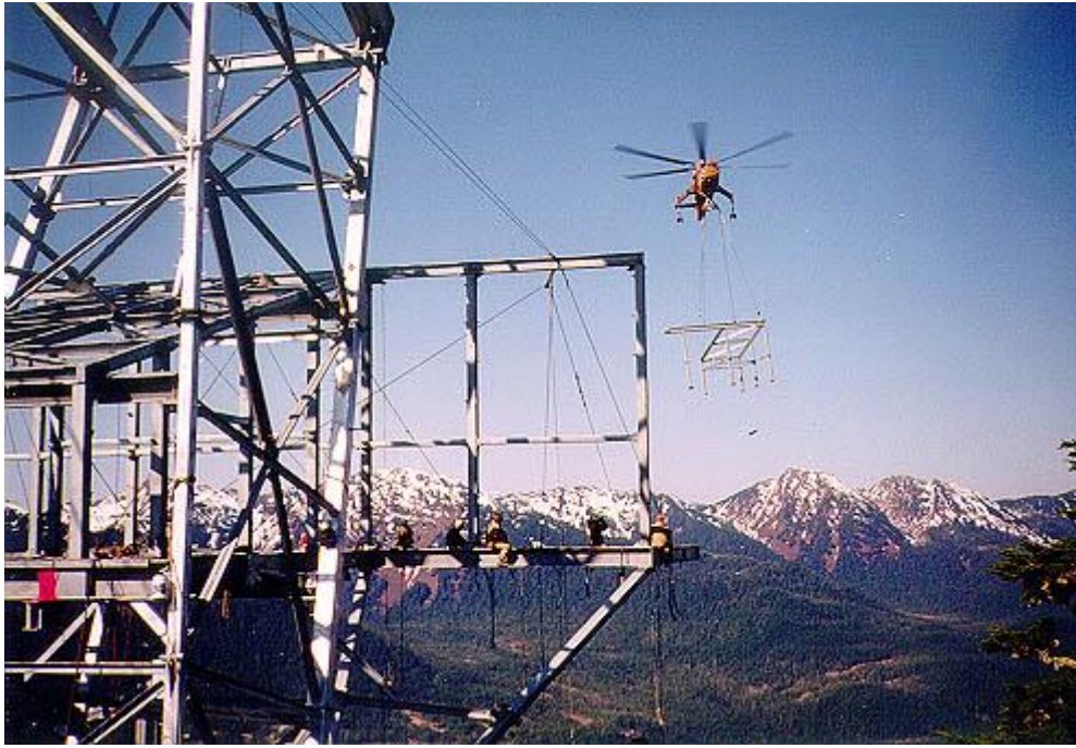
Structural steel can be slung into place by the Aircrane with precision and control unmatched by any other aircraft.
