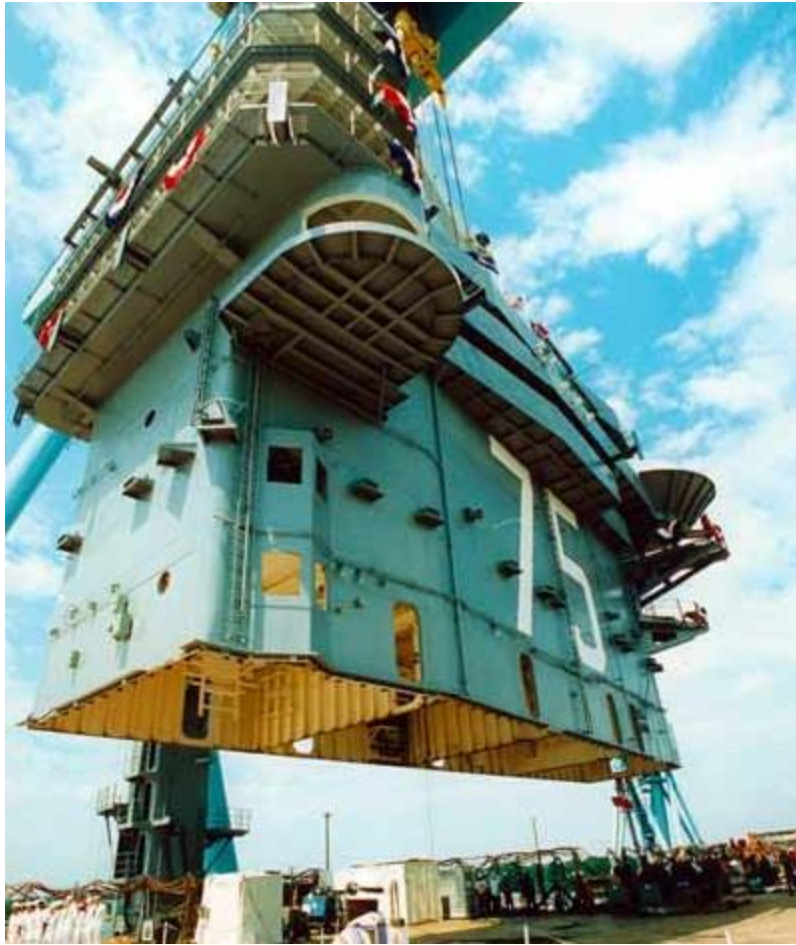
Photo courtesy U.S. Navy Lowering superlifts into position on the USS Harry S. Truman
