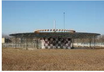
D-VOR (Doppler VOR) ground station, co-located with DME.
