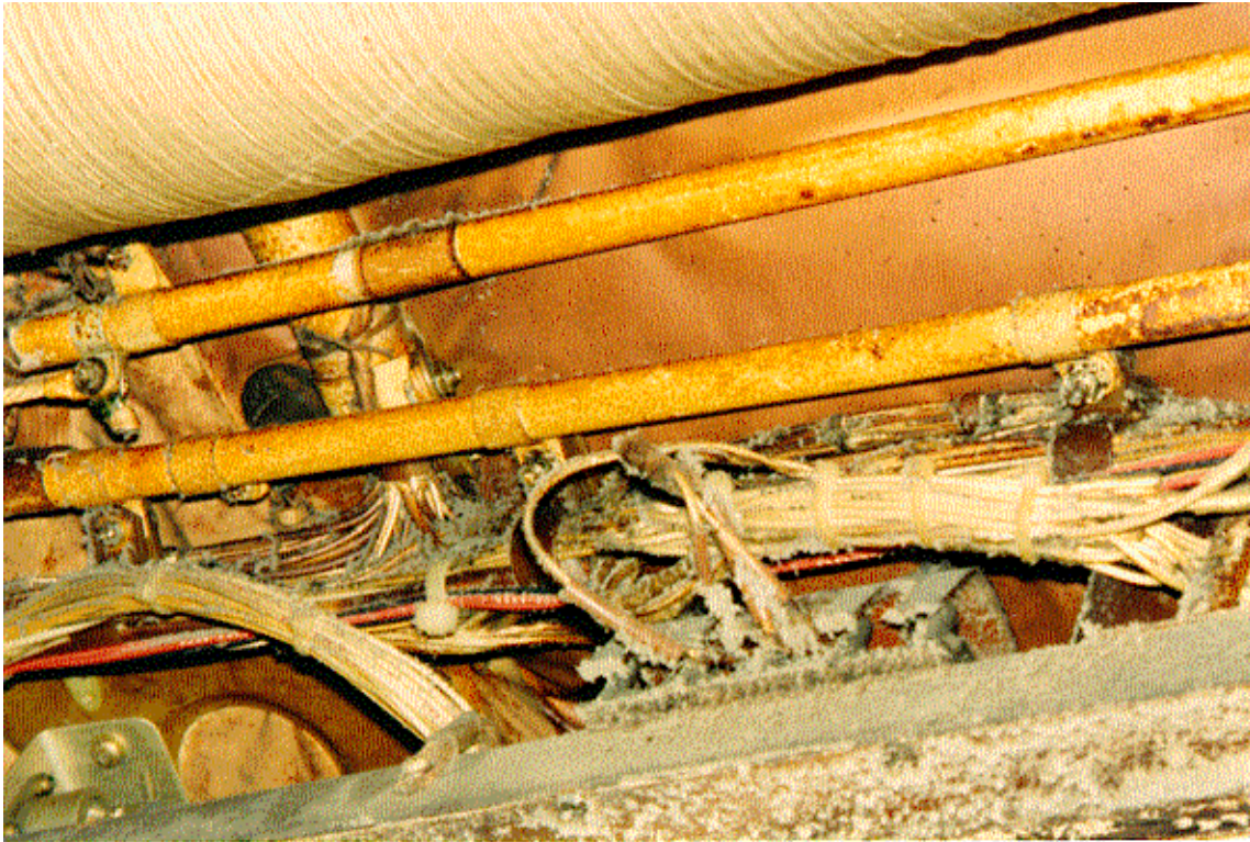
FIGURE 3-1. DUST AND LINT ACCUMULATION IN THE CROWN AREA
